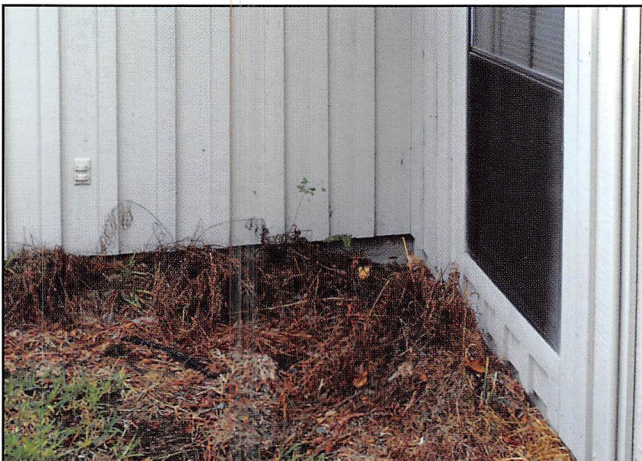
Inside corners can harbor embers.
