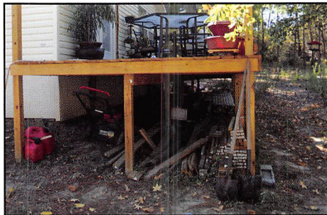
Embers landing on this wood could set your deck on fire.
