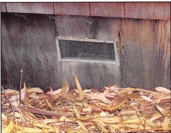
Combustible material like this mulch, near skirting or siding, leaves the home unprotected, even with screening in place. Photo by Institute for Business and Safety Research Center.
