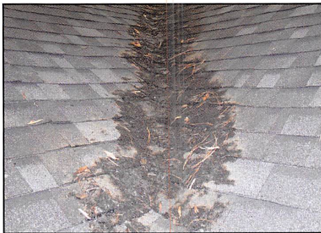
The pine needles on this roof burned, but the Class A roof did not. Photo by Institute for Business and Safety Research Center.
