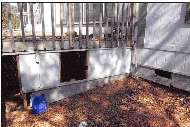
The flammable skirting under this deck, along with mulch, could easily lead flames to the deck and home.
