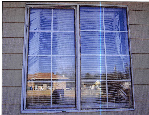
Radiant heat melted the interior blinds.
