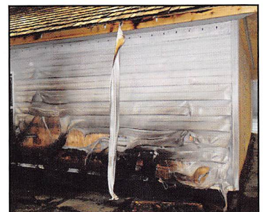
This vinyl gutter melted from heat, exposing the wood and roof edge to embers and direct flame. Photo by Institute for Business and Safety Research Center.
