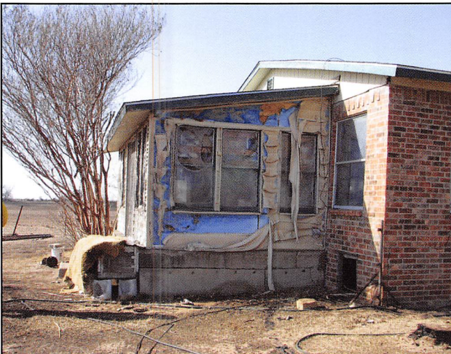
The vinyl siding and window frame on this home melted when exposed to radiant heat.
