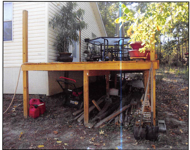
Materials under this deck could easily catch the home on fire.
