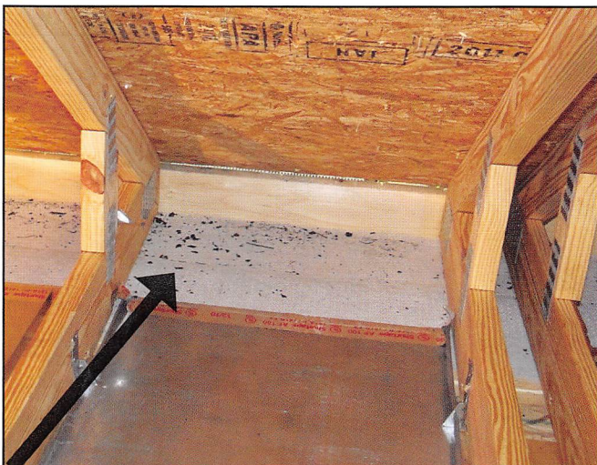
Without roof edge flashing, embers can enter into the attic. Photo by Institute for Business and Safety Research Center.
